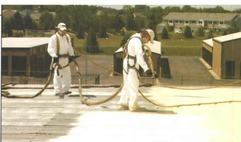
SPF can be applied to a variety of surfaces, including metal decks.
