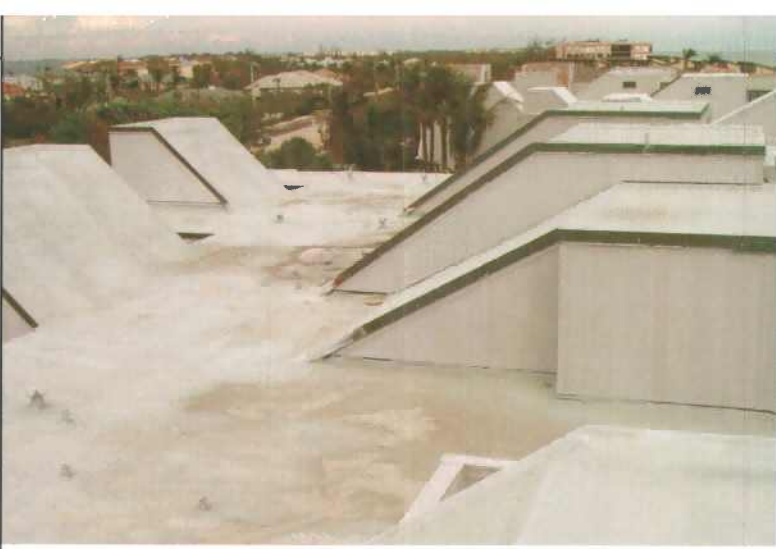
After direct hits from two severe hurricanes (Francis and Jeane) in Southern Florida, this SPF roof shows no damage from the storms.
